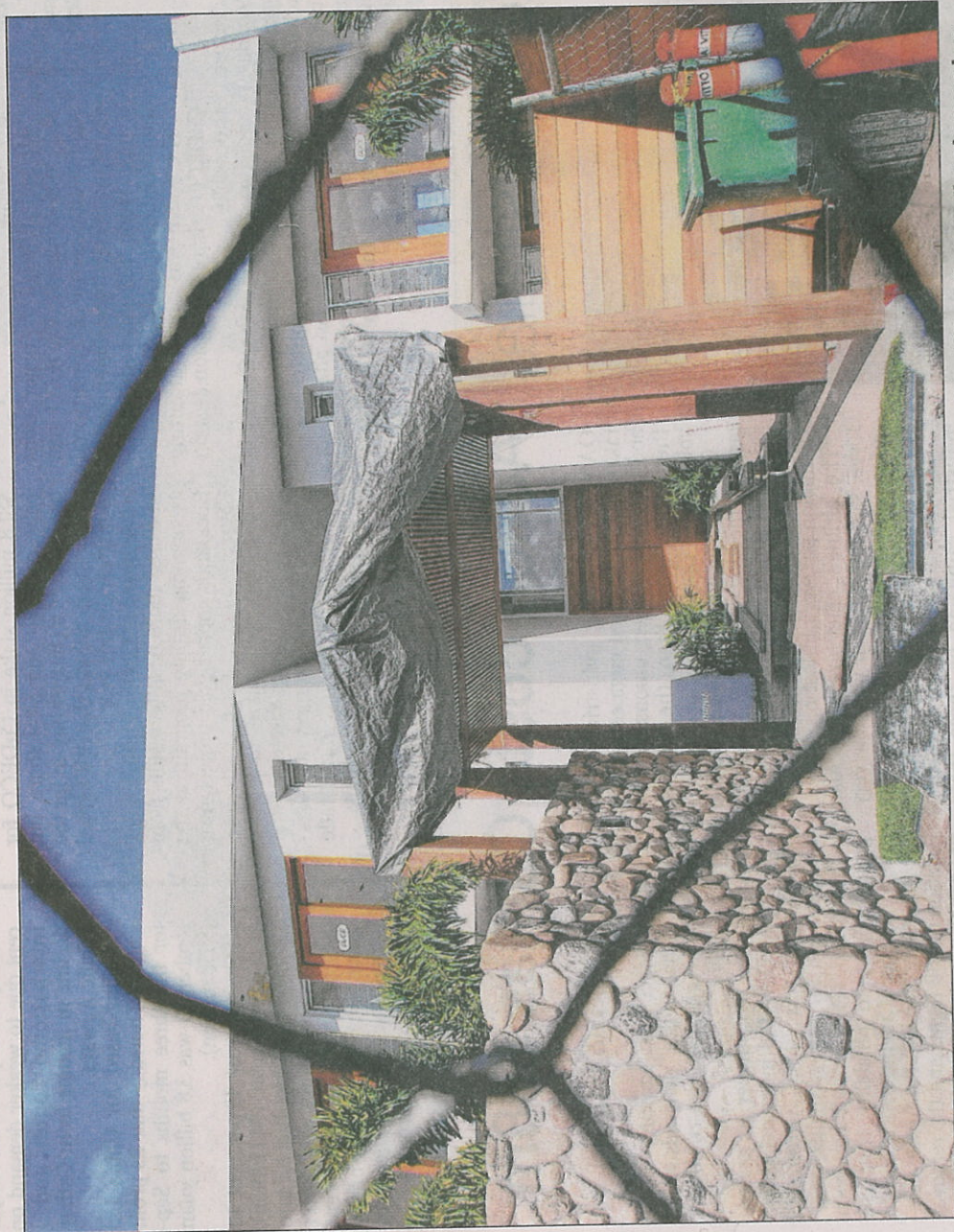
Work on this Regatta Parade, Southport, house has stopped for the second time as Vitto Ulliana Constructions is wound up
